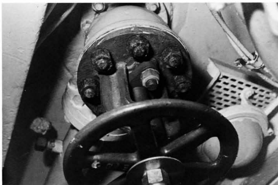
Figure 4. Steel Fastener Corrosion
