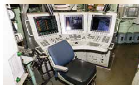
Figure 3. The Integrated Machinery Control System console designed for the Halifax -class frigates.
