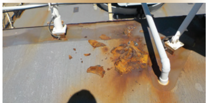
Corrosion – Bridge Top
