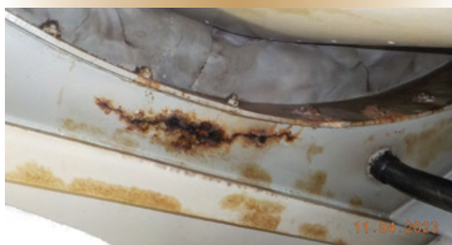
Corroded through deck
