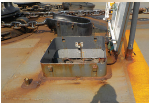
Corrosion – Hatch Coaming
