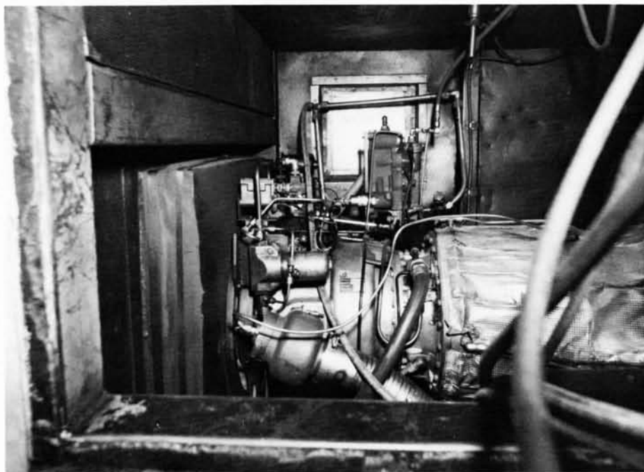
Figure 2. The existing acoustic enclosure in the Tribal-class destroyers.
