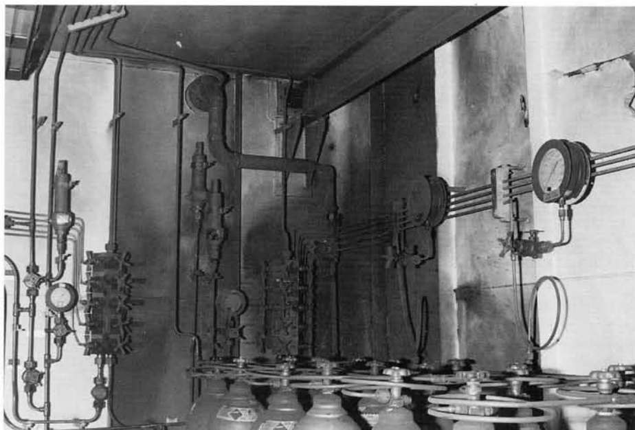
Fig. 1. The fire-damaged flask stowage compartment on board the diving-support ship HMCS Cormorant .
