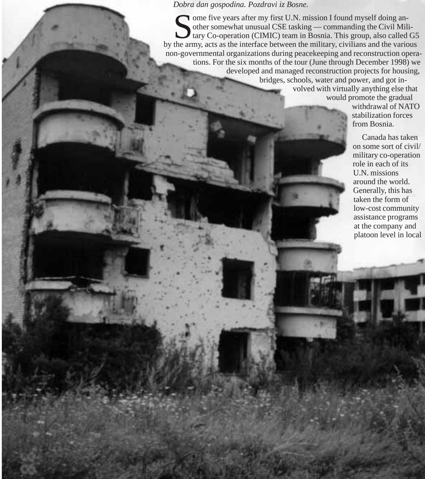
A destroyed apartment block. Note the numerous small-calibre bullet holes, and the holes from larger-calibre rounds on the side and front walls. This building is salvagable. (All photos courtesy of the author)
