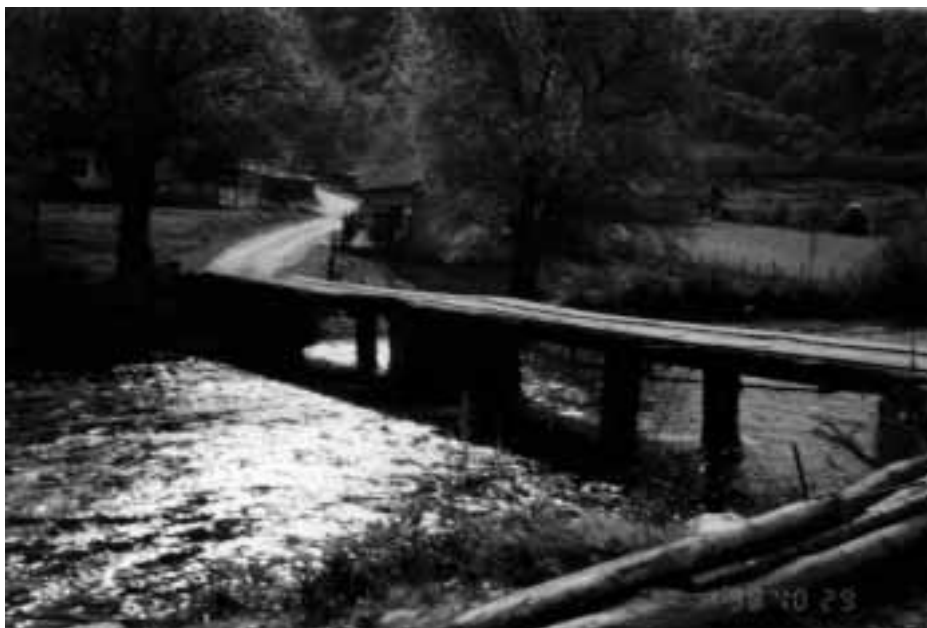
Heavy trucks crossed this small bridge over the Ribnik River daily. The bridge was later reconstructed.
