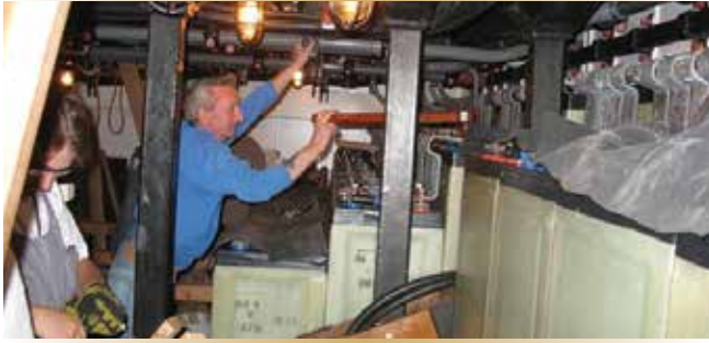
Tight work. A technician fits a lifting top onto a battery cell prior to its removal.
