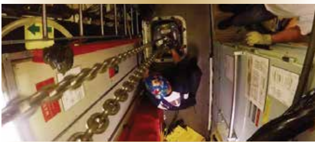
A healthy battery cell is lowered through a hatch on board Chicoutimi .
